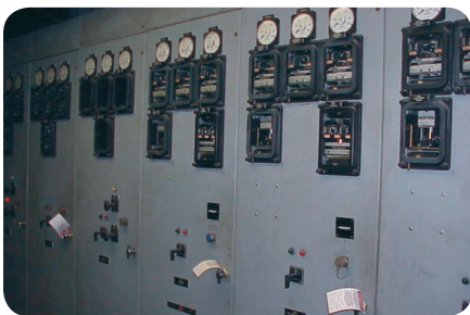
Fig. 1: Row of MCCs with installed EP-1000s.
